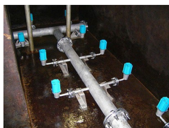
Vehicle factory Circulating water pit Putrefaction prevention and water purification February 2009
