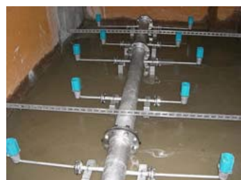
SHIMADZU CORPORATION Head office Kitchen wastewater treatment pit Water purification and deodorization September 2007
