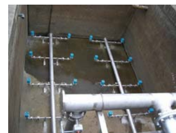
Fixed route bus storage yard Car wash wastewater treatment pit Water purification and putrefaction prevention December 2008
