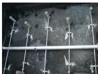
Fixed route bus storage yard Car wash wastewater treatment pit Putrefaction prevention and water purification July 2008
