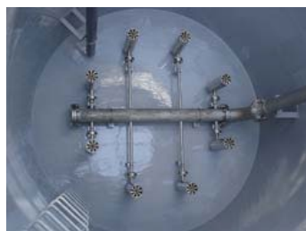
Food plant Wastewater treatment pit Water purification and putrefaction prevention February 2009
