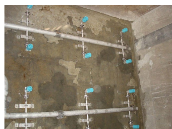
Food plant Wastewater treatment pit Water purification and putrefaction prevention January 2009
