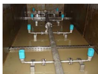
Truck manufacturing plant Circulating water pit Putrefaction and deterioration prevention October 2008
