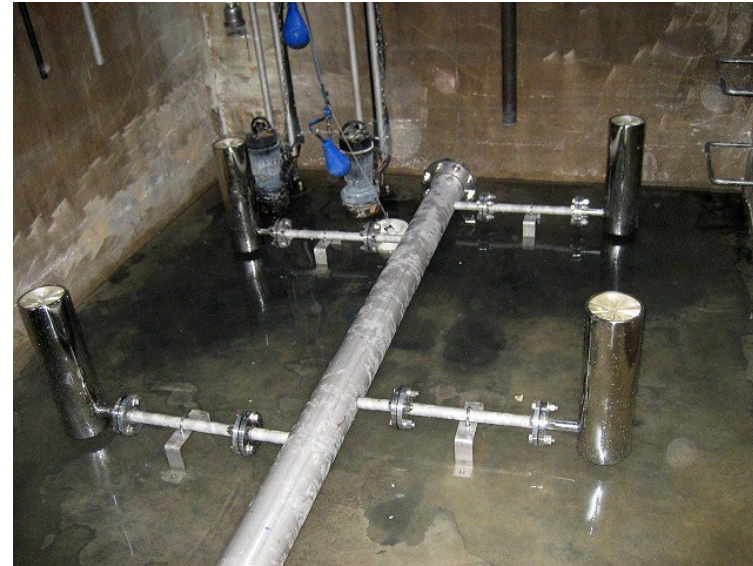
Treatment tank internal piping
