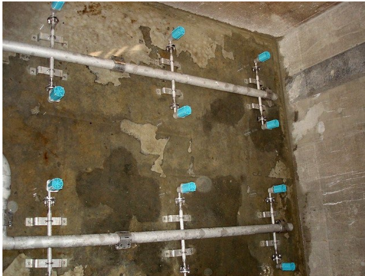
Adjustment tank internal piping
